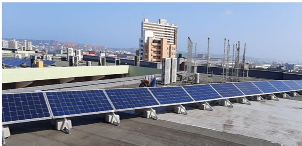
Fig. 1 A roof-mounted solar PV at DUT
